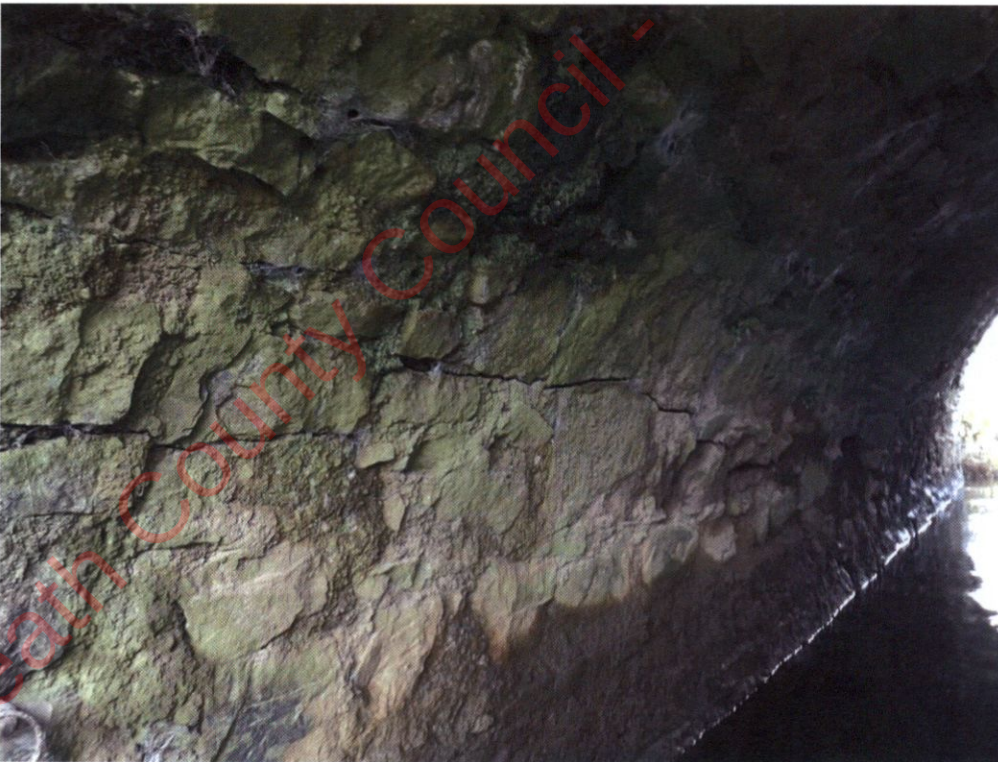
Photograph B-22 – Transverse crack to the bottom of arch barrel 1 above the north abutment
