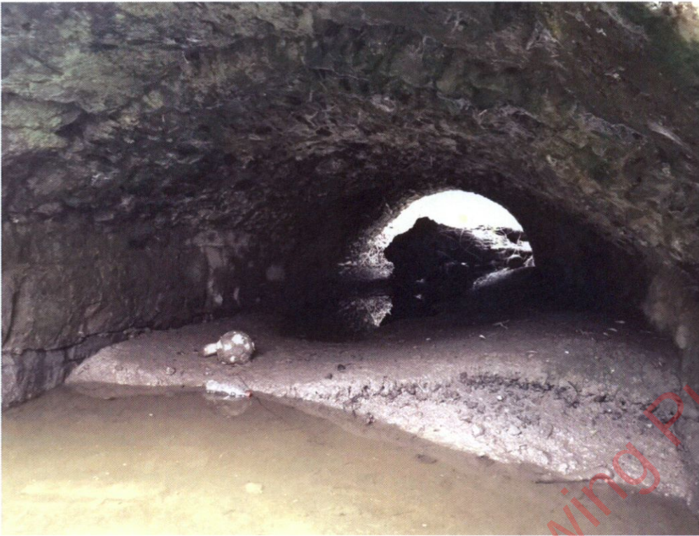
Photograph B-29 – Arch barrel 7 with water ingress and minor pointing loss evident and debris located at the west elevation with a change in the arch profile evident
