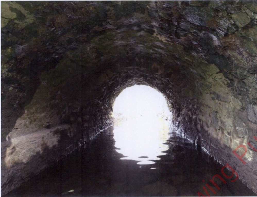
Photograph B-27 – Arch barrel 5 with water ingress and minor pointing loss evident with a change in the arch profile evident
