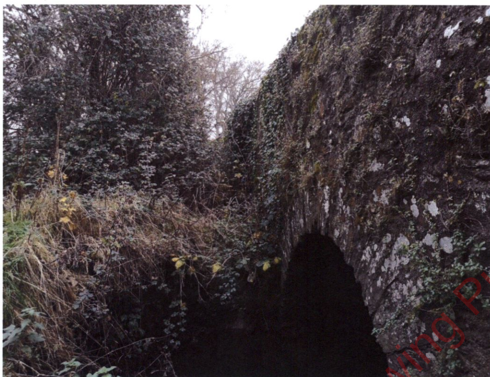
Photograph B-9 – SE embankment with overgrown vegetation evident
