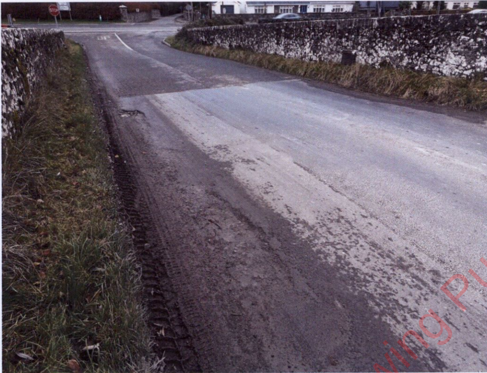
Photograph B-3 – Area of depression to carriageway surface above pier 3. Note tie into R150 road surfacing above arch 3.
