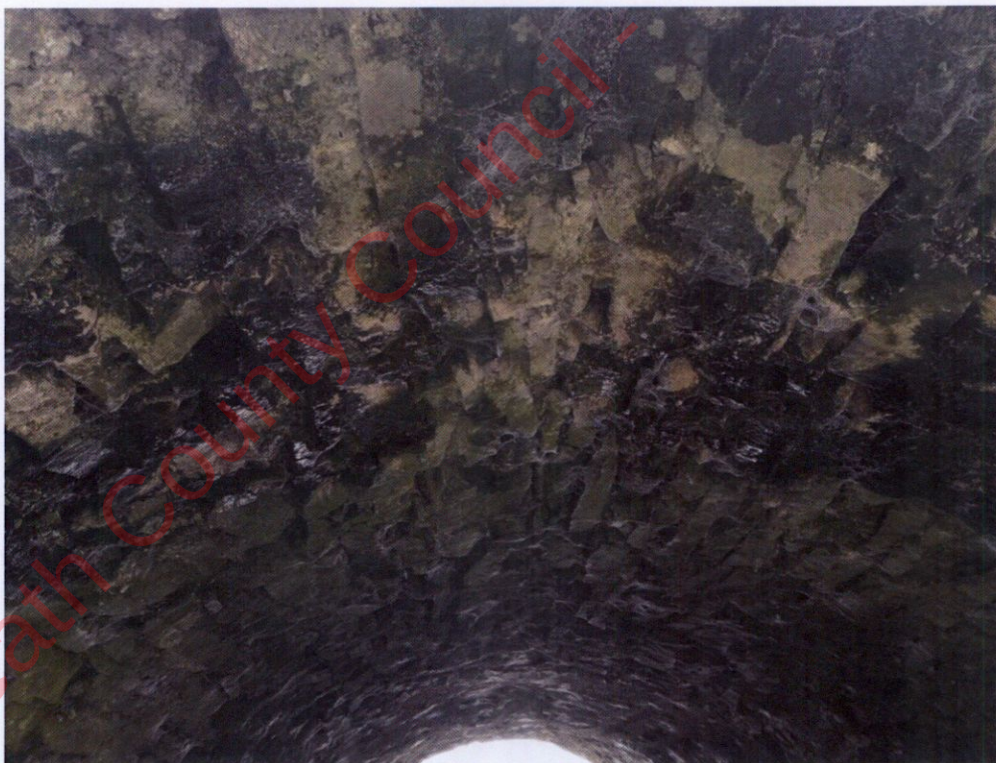
Photograph B-24 – Arch barrel 2 with pointing loss, minor masonry loss and water ingress evident
